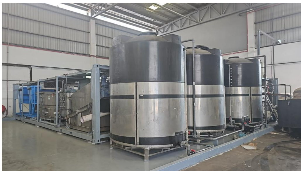
Photo of hazardous waste storage
